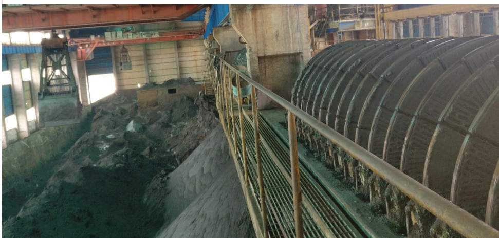
Flowrox Ceramic Disc Filter performs extremely well in copper tailings filtration.
